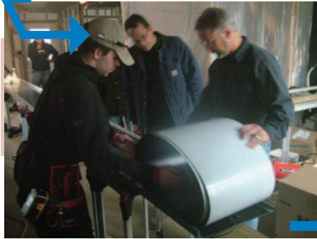
A trained metal roofing contractor installs the BIPV laminate directly onto a metal roof panel at the job site.
