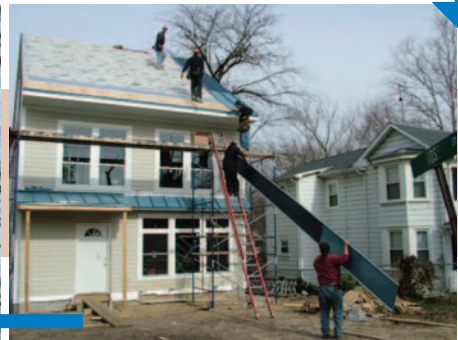
The metal roof panel are installed by a trained metal roofing contractor.
